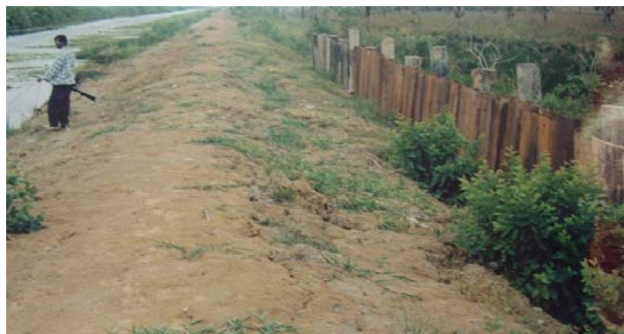
Photo 11: EDWC East Dam downstream slope failure
