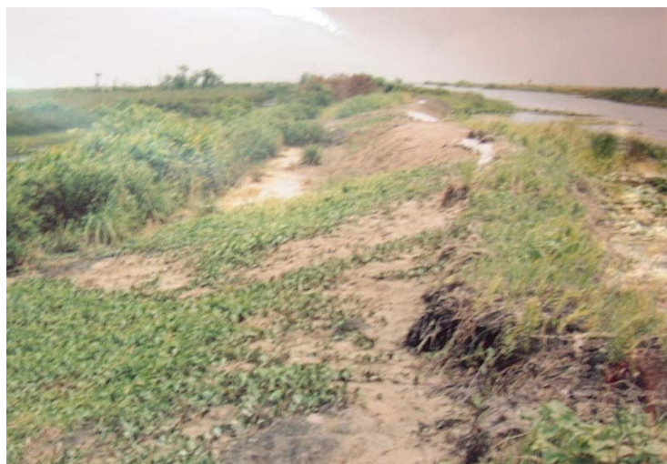
Photo 6: EDWC poor condition of EDWC North East Dam: Deteriorated Crest
