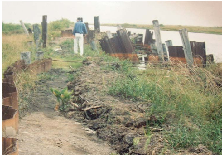
Photo 4: EDWC North East Dam location needing urgent repairs
