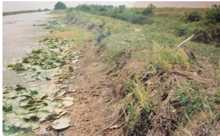
Photo 5: EDWC poor condition of EDWC North East Dam: Upstream slips
