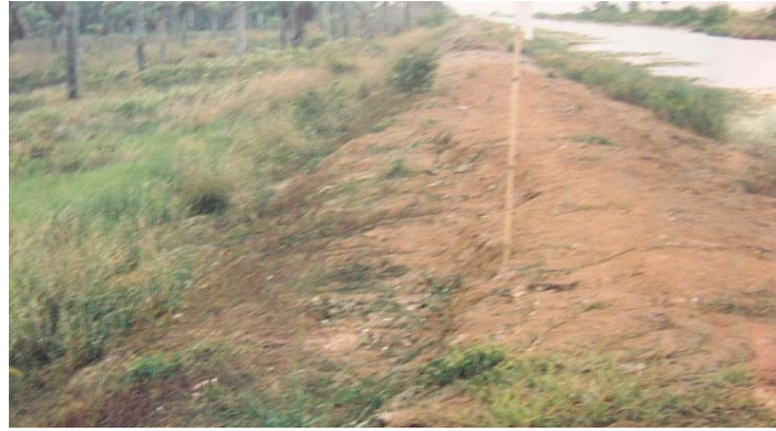
Photo 10: EDWC East Dam downstream slope failure
