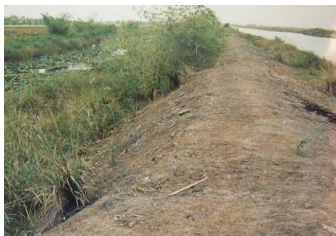
Photo 9: EDWC North East Dam proximity of borrow trench (flooded)
