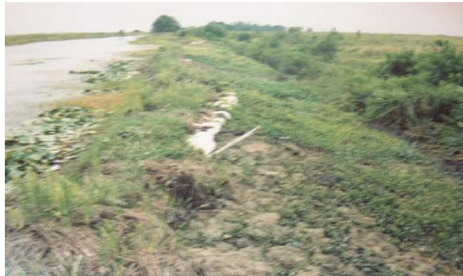
Photo 7: EDWC poor condition of EDWC North East Dam: Damaged Crest
