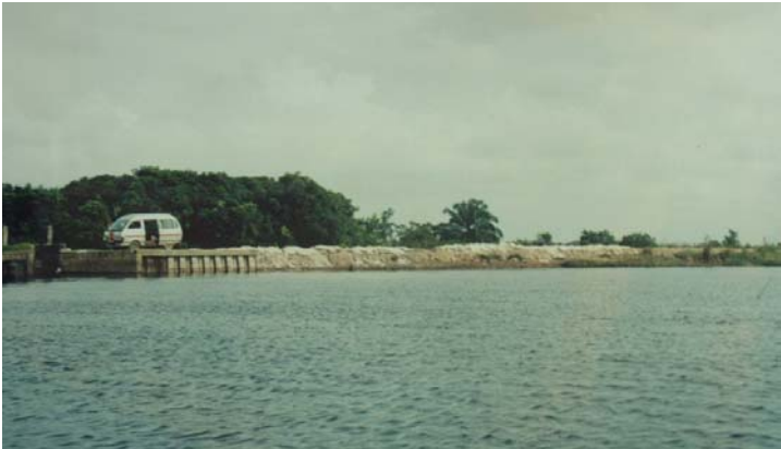
Photo 17: Boersarie East Dam broken sand bags
